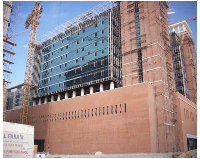
CLIENT: First Gulf Bank CONSULTANT: Bainona Consulting Engineering CONTRACTOR: Al Fara'a General Contracting Co. L.L.C
